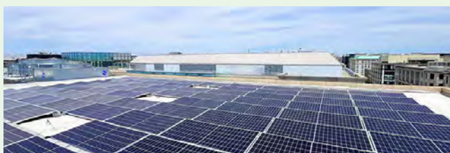
The rooftop solar array, hidden from view, but generating clean energy that can be experienced throughout the building
